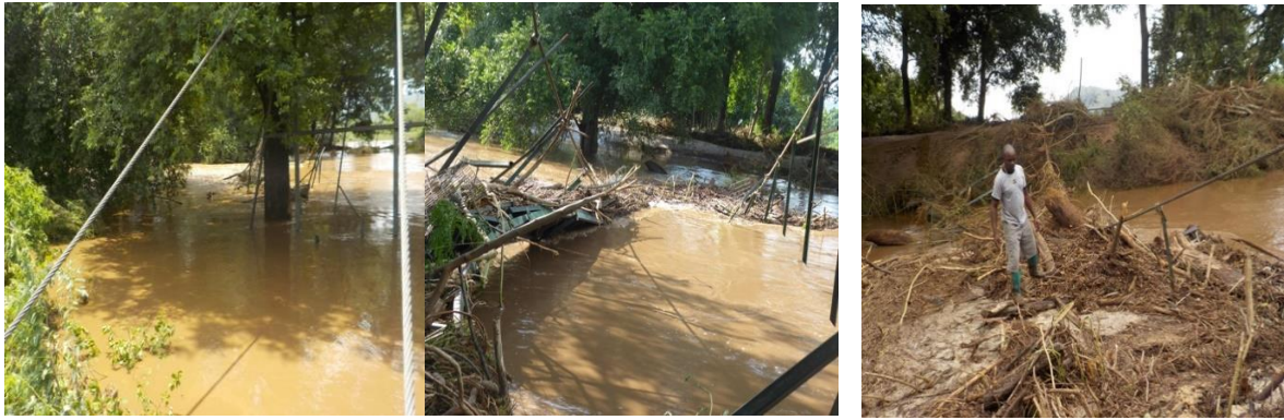
Figure 3: The foot bridge during the flood and being assessed after the flood
